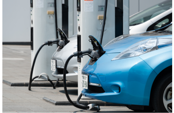
Electric vehicles using charging infrastructure
